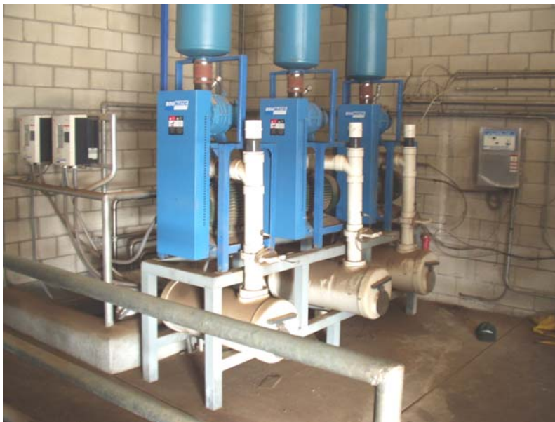
Figure 1-7. VFD vacuum pumps on California dairy
