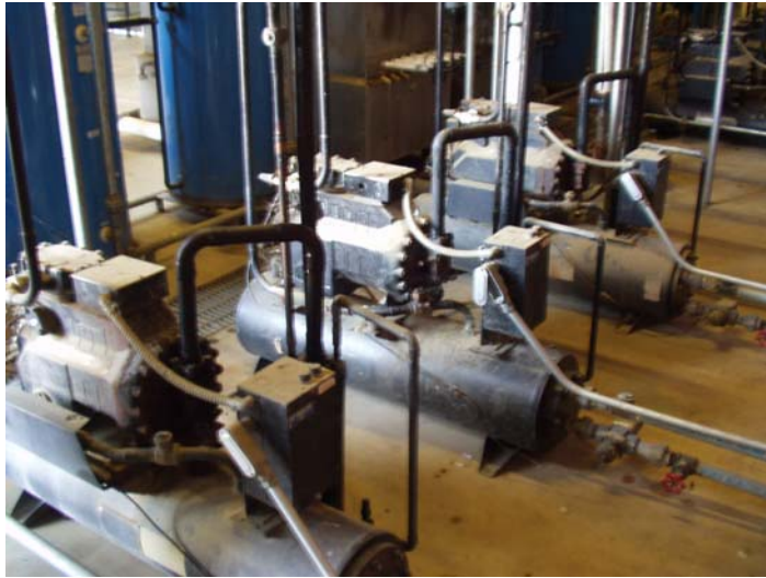
Figure 2-6. Water-cooled condensing units with accessible hermetic compressors
