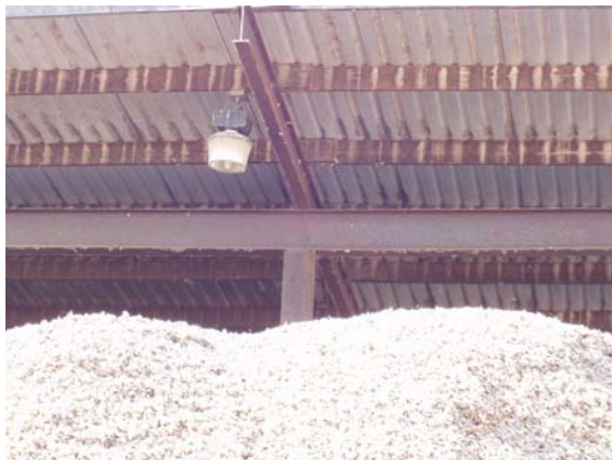
Figure 3-9. High pressure sodium fixture in commodity storage shed
