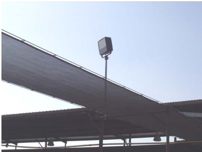
Figure 3-8. Example of 1,000 W floodlight for feeding corral lighting
