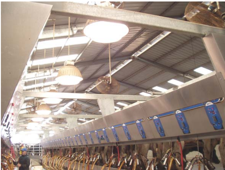
Figure 3-2. Example of metal halide milking parlor pit lighting
