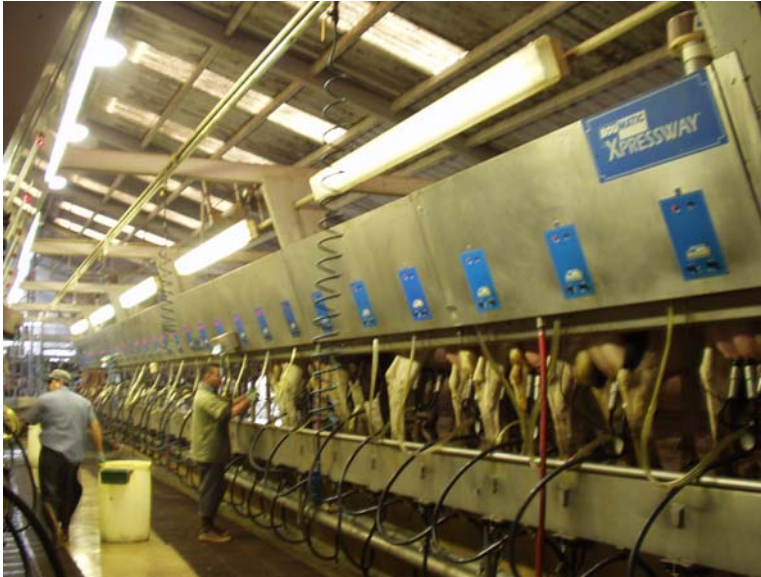
Figure 3-1. Example of fluorescent milking parlor pit lighting
