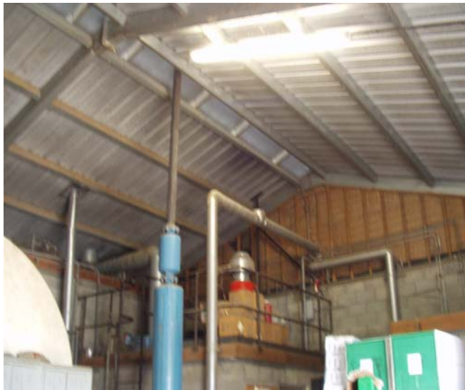
Figure 3-5. Fluorescent lighting in a utility room
