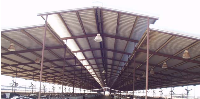
Figure 3-6. Example of metal halide lighting in a dairy cattle confinement feeding barn
