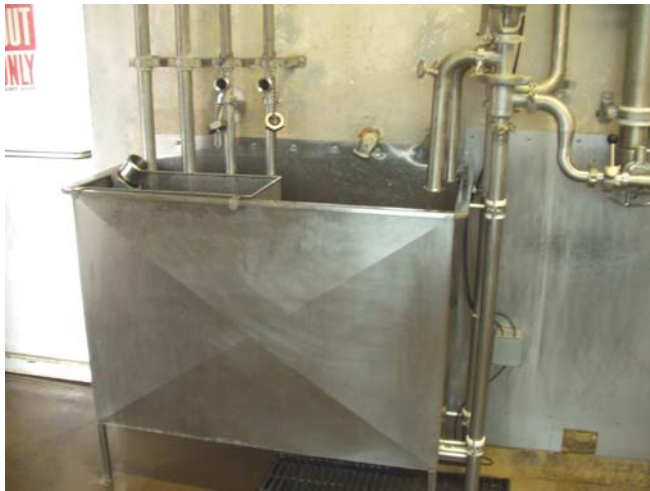
Figure 5-8. Wash sink on California dairy
