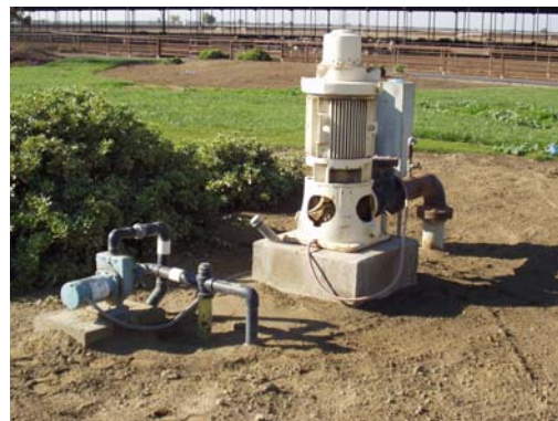
Figure 6-4. Typical well water supply pump pumps on California dairy
